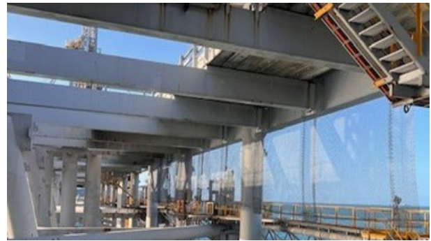
Figure 11 Mesh installed across several bays has a low impact on visibility for all end users – BMA, (2024)
